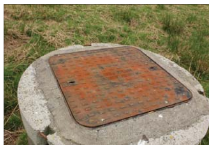
Plate 39 - Round concrete drainage access structure with square 'Clark Drain Pedestrian' cast iron cover
