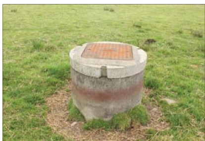
Plate 37 - Round concrete drainage access structure with square 'Clark Drain Pedestrian' cast iron cover
