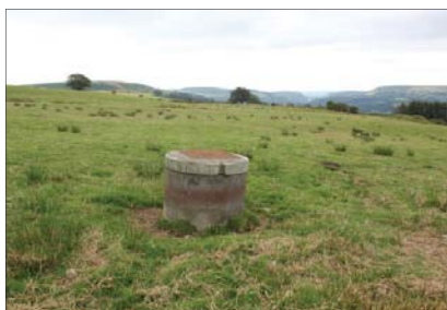
Plate 38 - Round concrete drainage access structure with square 'Clark Drain Pedestrian' cast iron cover
